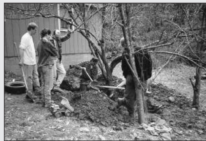
Trying to clear a blockage in a sewage system
