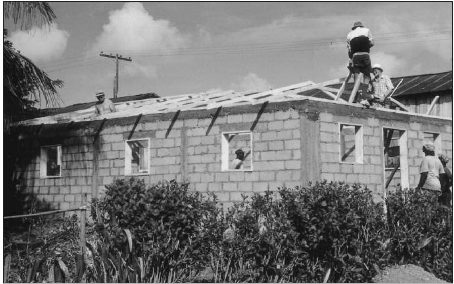
Construction of the simple, concrete-block building goes on under the hot sun.
