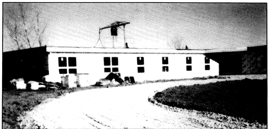
One wing is now under the roof. To the right the new main entrance
